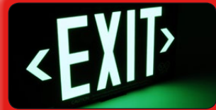
SECURITY SYSTEMS AND EMERGENCY LIGHTING
